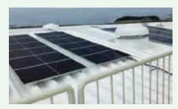
Solar power generation equipment installed at the Oppama Plant
